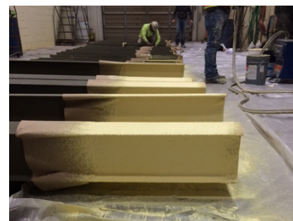
Tnemec’s thermal insulating coating, Aerolon, was applied to steel beams for a Pennsylvania student union to mitigate thermal bridging and limit condensation within the building.
