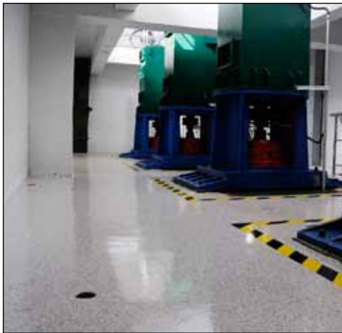
Tnemec's Series 224 Deco-Fleck, a flake-filled polyamine epoxy floor topping, was the solution to the flooring needs at the Pudong Waigaoqiao No.3 Pump Station.
