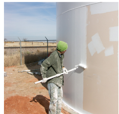
A fast-curing product was needed for the Alabama Avenue ground storage tank, which is why Series 740 UVX was chosen as the exterior topcoat.
